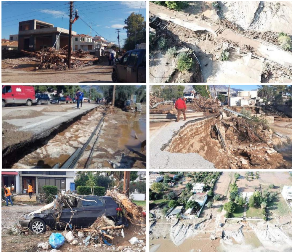
Figure 3. Damages by the flood of 2019 to infrastructure, road networks, and the coastline of the Kineta area [55–57].
