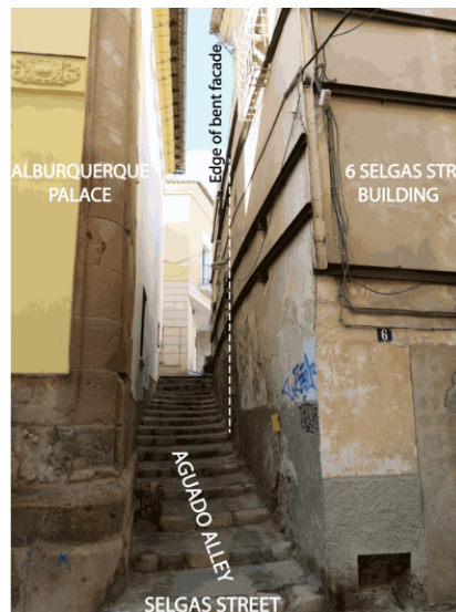
Figure 11. View towards the NW of the 6 Selgas Street building with the bent Aguado alley facade. The Albuquerque palace on the left part of the photograph also shows a bent Aguado alley facade, and the Aguado staircase is deformed between the two facades (modified from García-Mondéjar et al. [23]).
