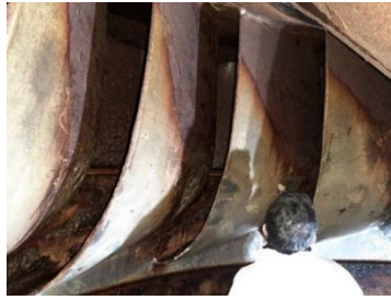
Figure 1. Existing runner of power plant.
